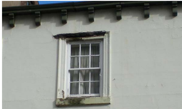
Fig 45. A neglected gutter spilling water onto masonry and window below.
