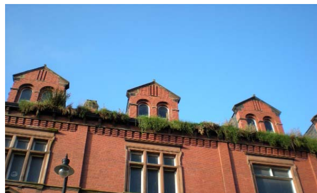
Fig25. Neglect of basic maintenance in the former Boustead's building, latterly Mood's Nightclub.
