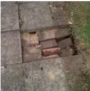
Entrance hole in paving
