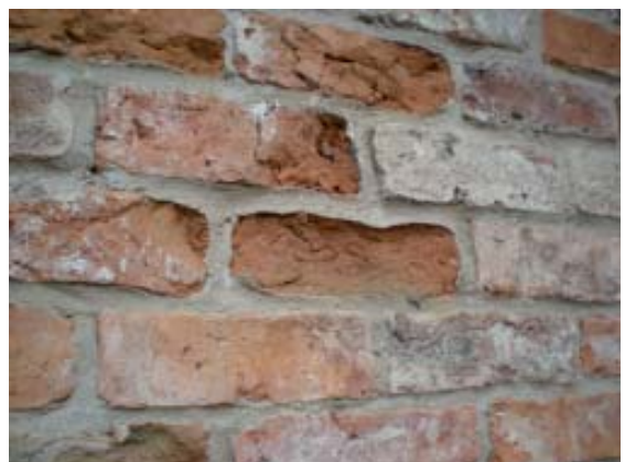
▲ Accelerated decay of bricks caused by inappropriate cement pointing
