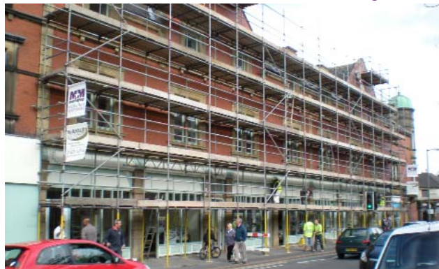
Fig 32. Great improvements to the appearance of Stanley Hall were made by McKnight's builders in 2011.
