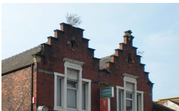
Fig 46. Buddleia growing in coping could eventually unseat the masonry unless removed.
