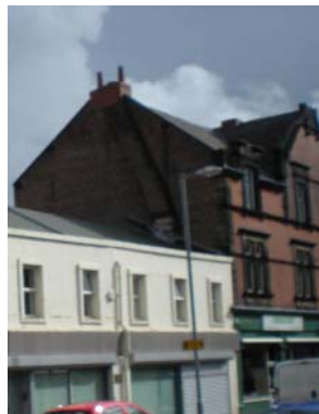
Fig 30. Truncated chimney stack to the Stanley Hall.
