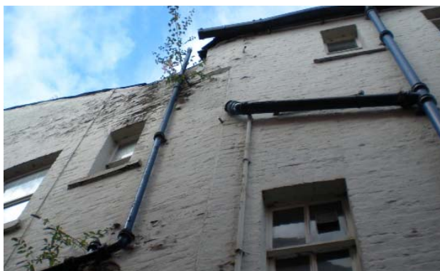
Fig 44. neglected maintenance of gutters leading to vegetation growth and likely damage to building fabric.
