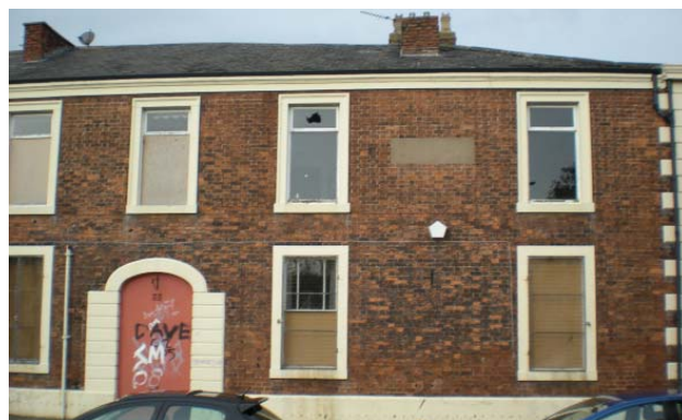
Fig 58. Unoccupied former surgery at Woodruffe Terrace, suffering casual vandalism.
